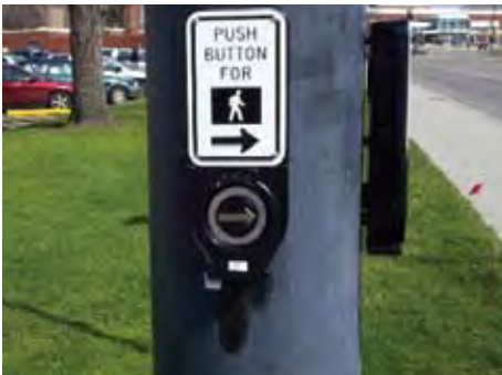
Accessible Pedestrian Signals
